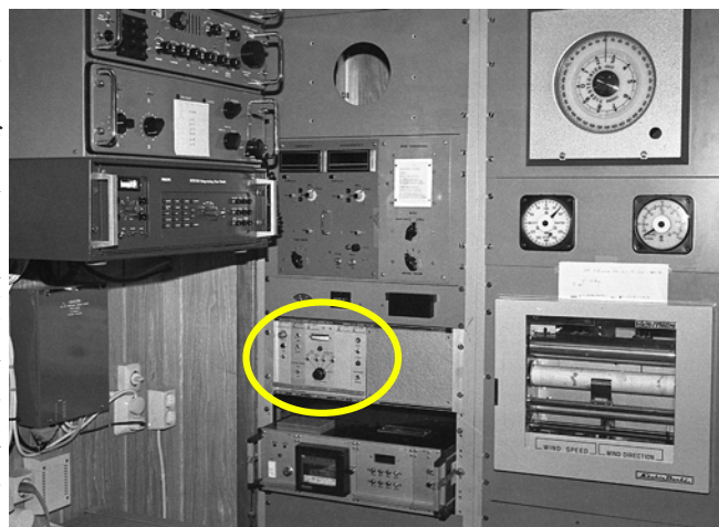
Metoccean and navigation instruments on the Norwegian weather ship Polar Front . The SBWR console is in the centre rack.
